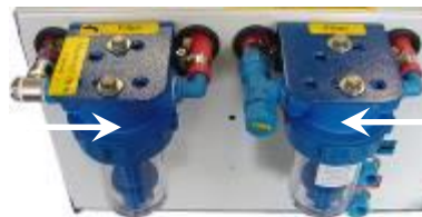
Cooling water filter
